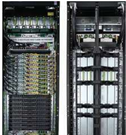
Figure 5. Meta's Catalina ORv3-HPR rack shown from the front (left) and rear. It delivers up to 140 kW/rack for next-generation AI workloads. Adapted with permission from Reference 5.
